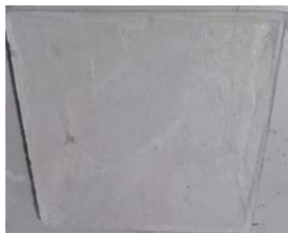
Concrete substrate with dusty surface
